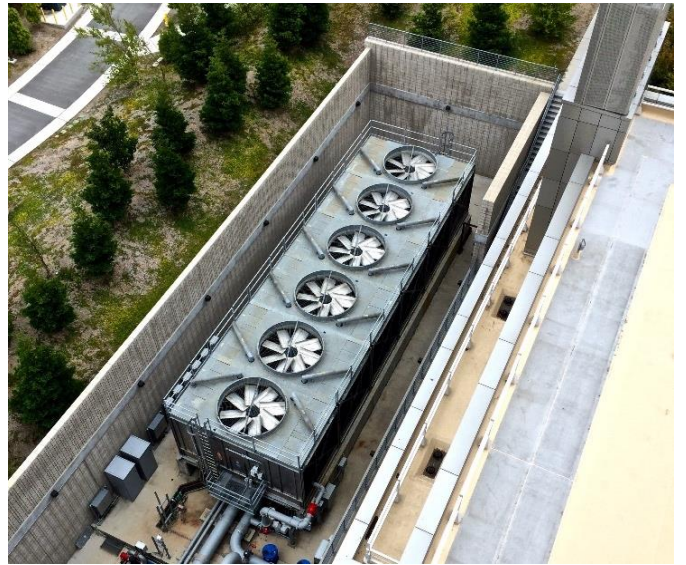
Figure 1: Image of Cooling Towers from the Hospital from which the Data Originates
